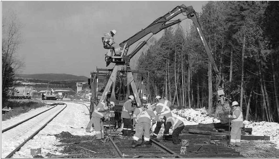
Workers from the Société du chemin de fer de la Gaspésie will be called upon to speed up repair work on the railway.
